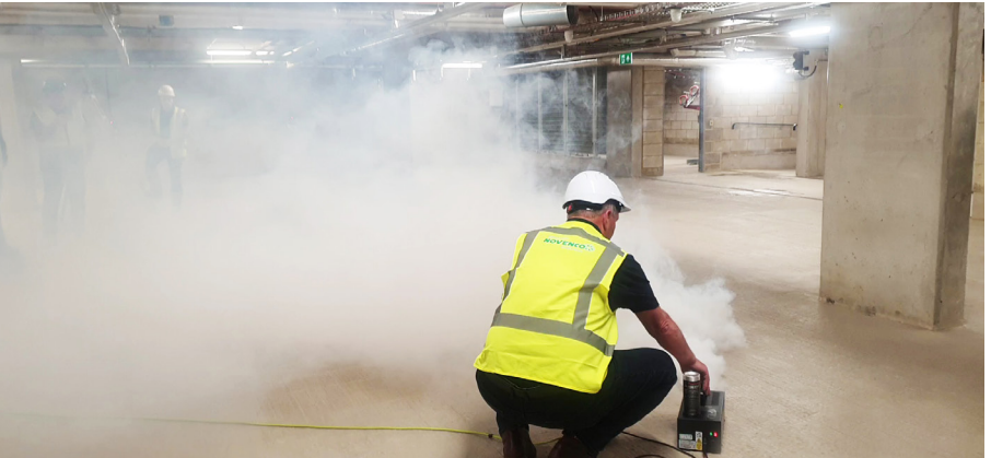
The NOVENCO’s smoke clearance system test in carpark
