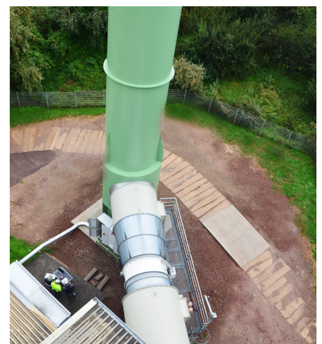
View on the new ventilation system from above
