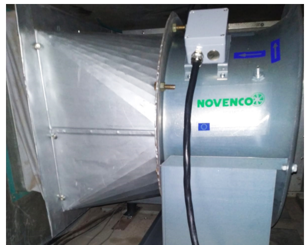
One of the 40 NOVENCO ZerAx EC+ fan installed at the DS Groups' headquarters as a plug-and-play easy retrofit
