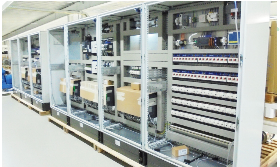
6 motor control panels for smart control of the whole car park ventilation system
