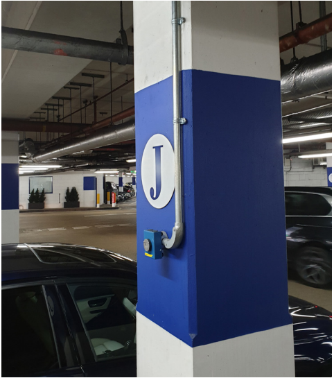
One of the CO detection heads within the car park
