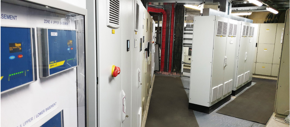
One of the main control panel rooms with the new 75kW extract fan variable speed drives
