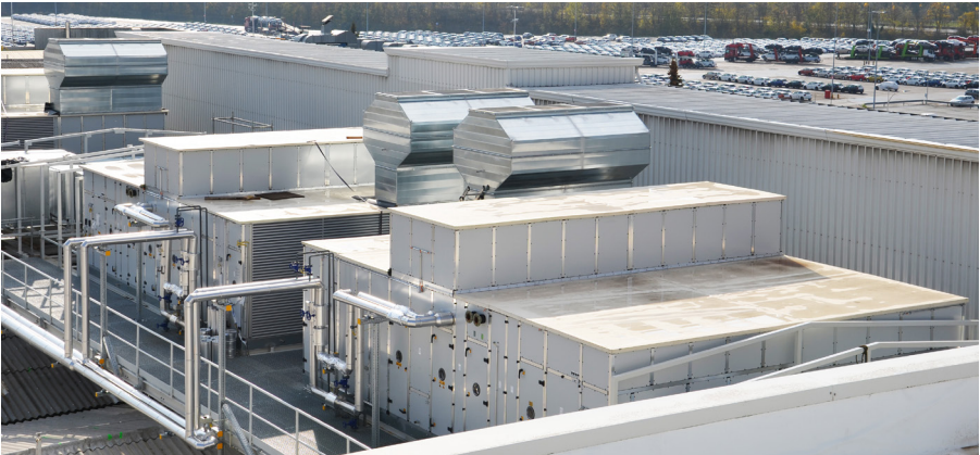
Three roof-installed AHUs, each with 60,000 m 3 /h
