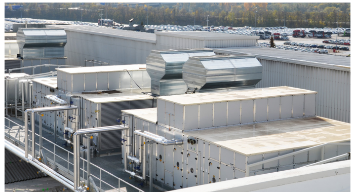
Roof-installed AHUs with ZerAx axial fan
