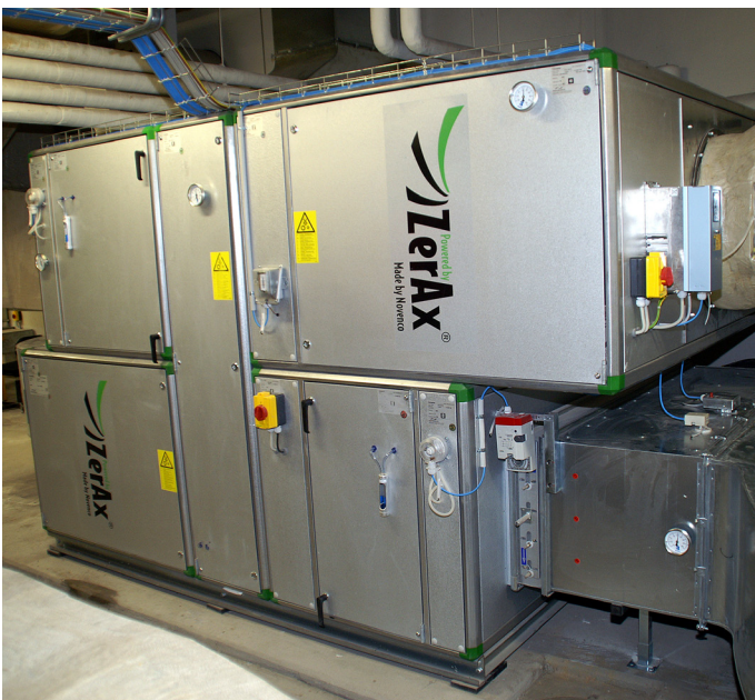
Air handling unit Climaster ZerAx® installed in Aarhus Concert Hall
