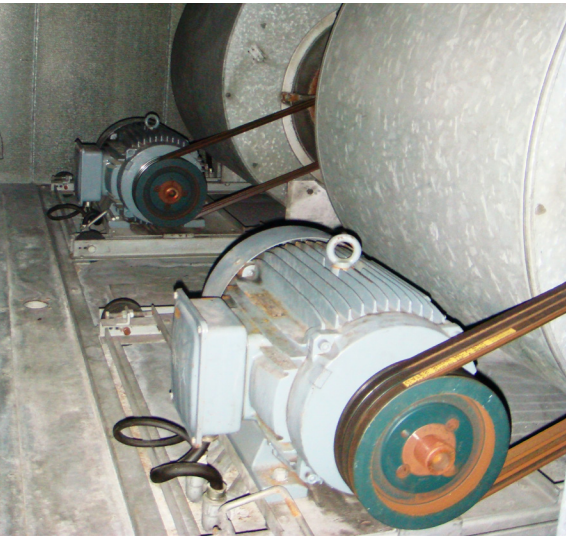
Old fans installed in the 1970's
