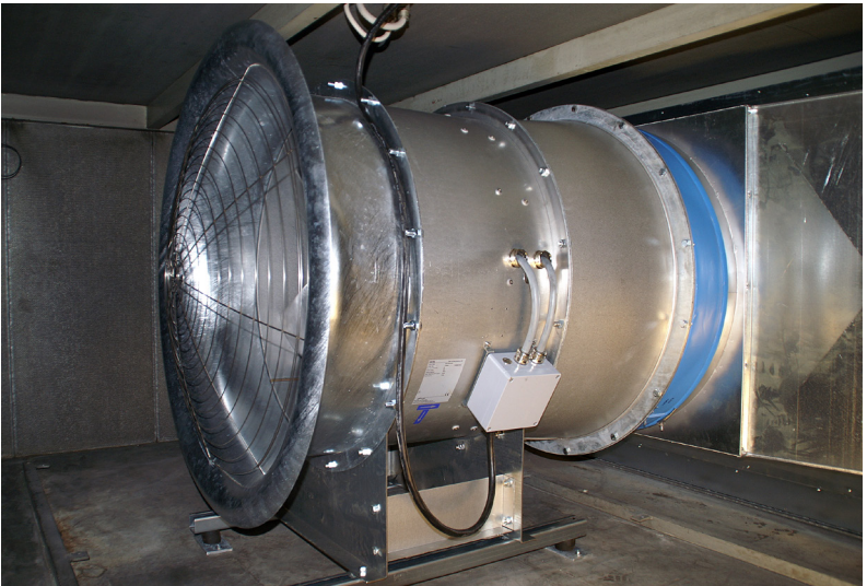
ZerAx® fans installed at the brewery in Fredericia
