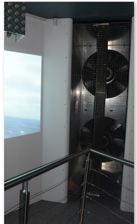
The fan array installed at The Port exhibition
