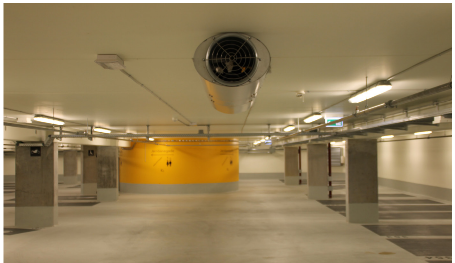
Installation with NOVENCO jet fan AUO
