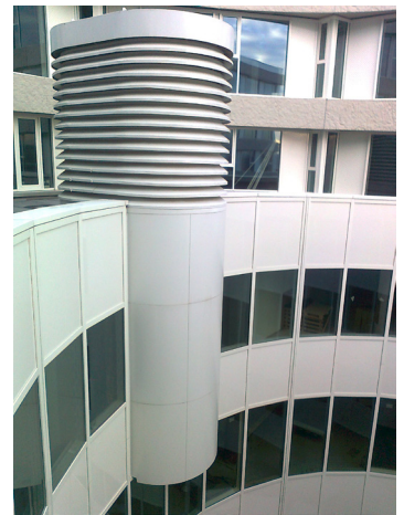
One of the fan exhaust towers
