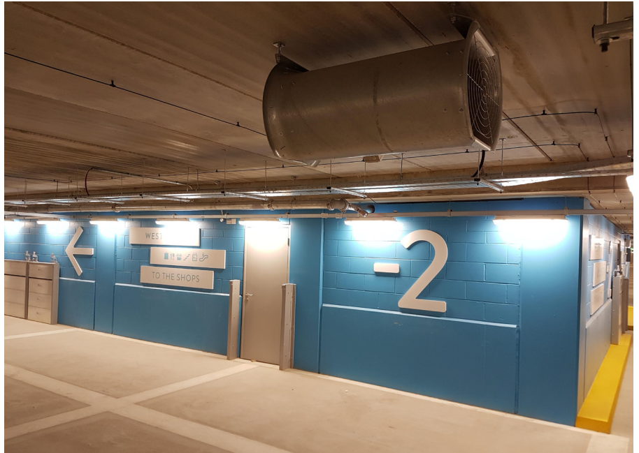
Westage Oxford's car park equipped in NOVENCO's ventilation system
